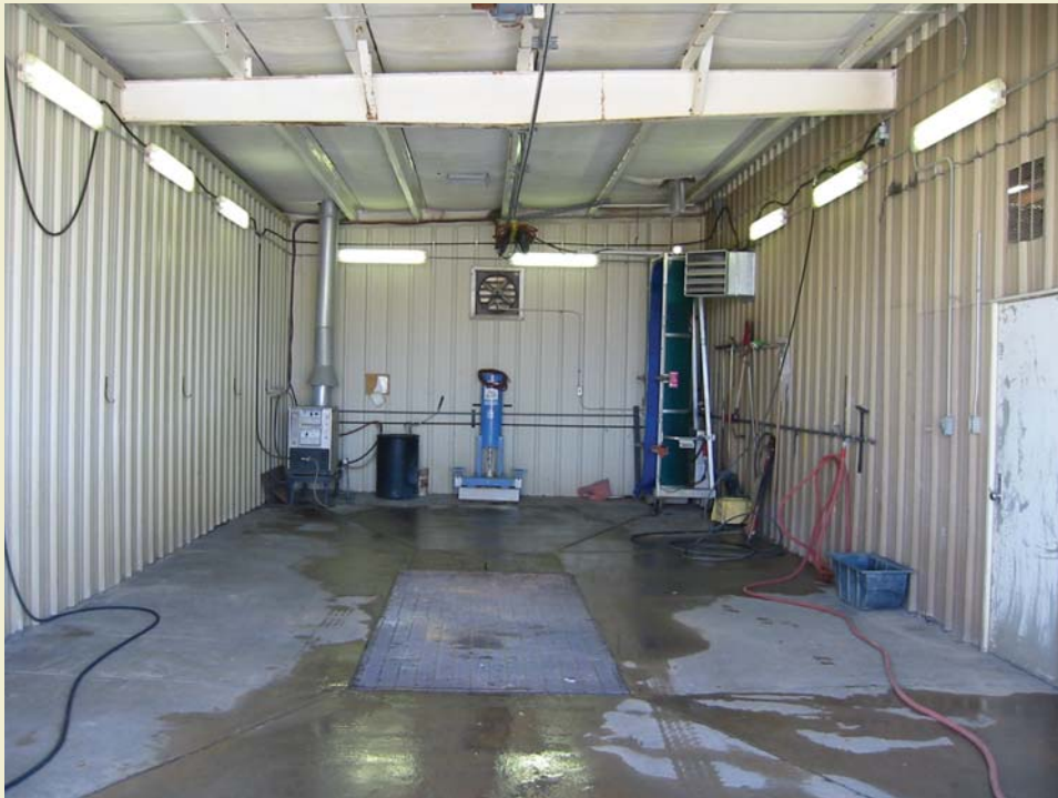
Floor drains in service bays might lead to a Class V (Five) Motor Vehicle Waste Disposal Well.
