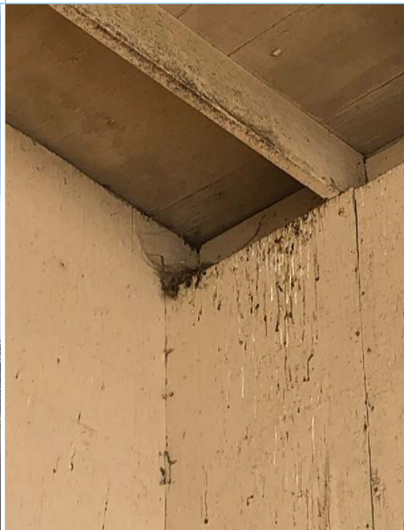
Photograph 16: Remnant bird nest inside barn.
