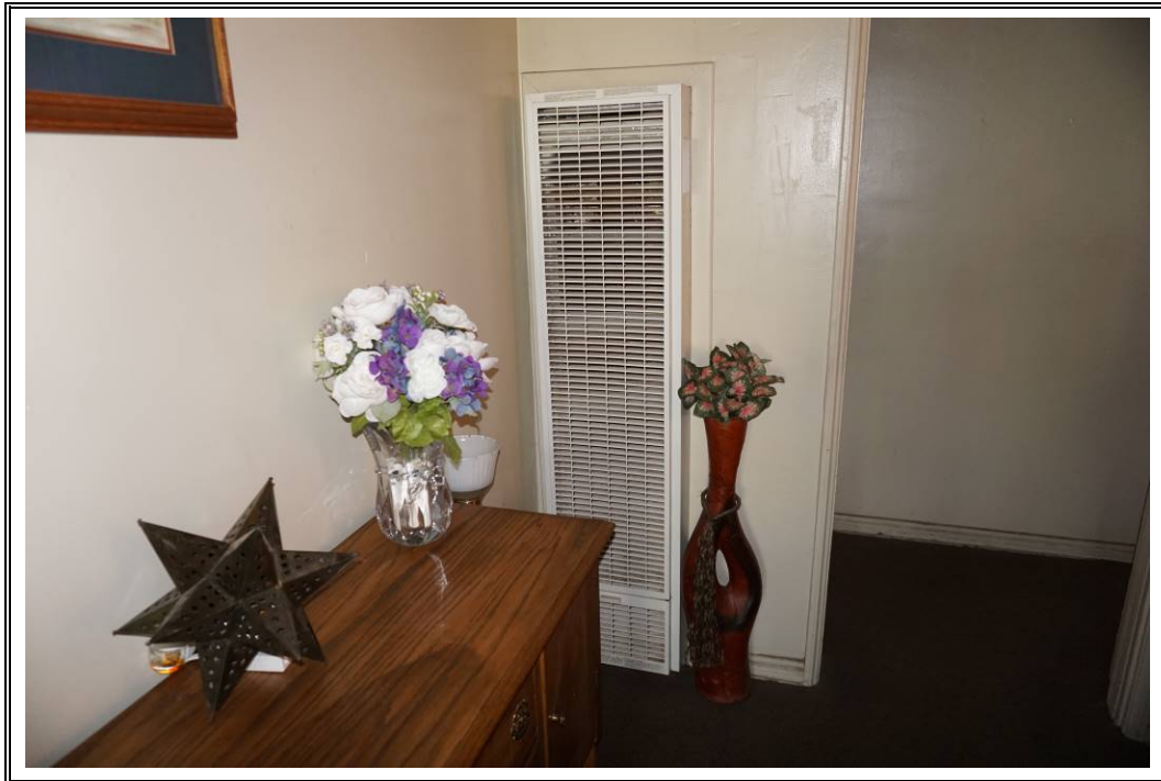
Photograph Number 39: View of wall-mounted natural gas heater within subject property dwelling interior (14557 Chandler Street).
