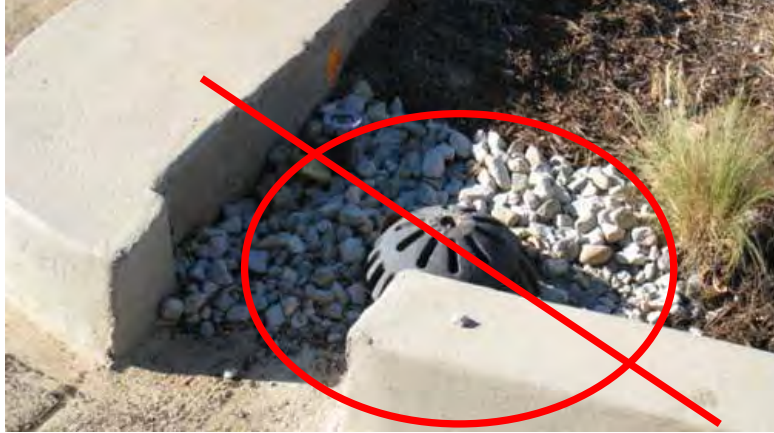
Figure 6: Incorrect Placement of an Overflow Inlet.
