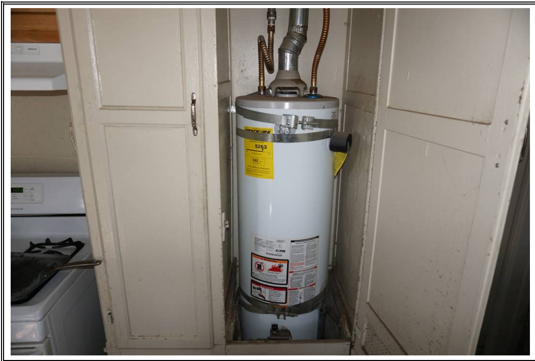
Photograph Number 38: View of natural gas hot water heater within subject property dwelling interior (14557 Chandler Street).
