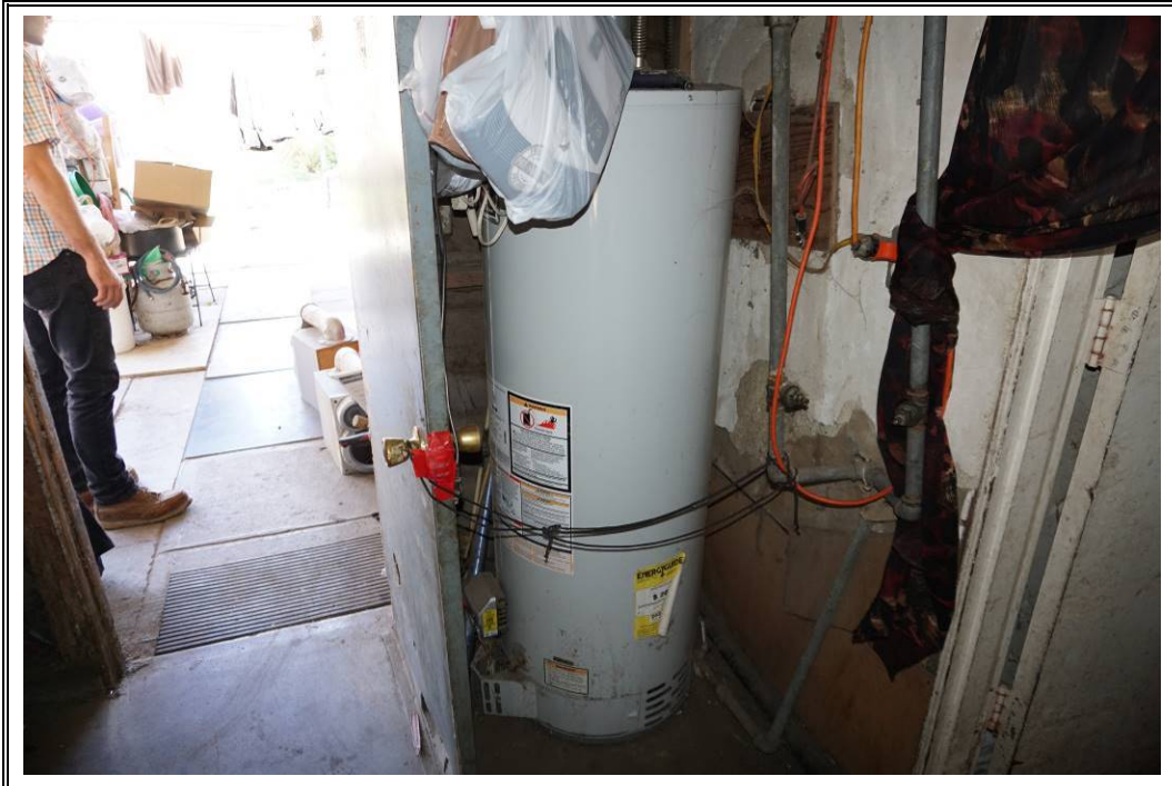
Photograph Number 47: View of natural gas hot water heater within subject property dwelling interior (14577 Chandler Street).
