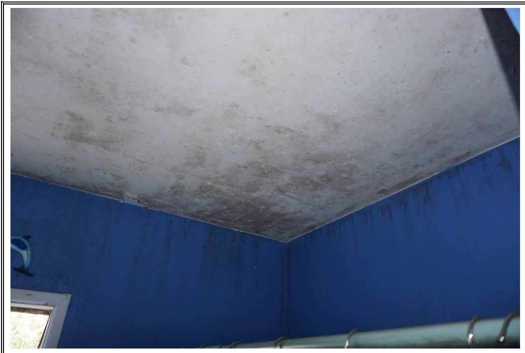
Photograph Number 34: View of mold/mildew growth within subject property dwelling interior (14555 Chandler Street).
