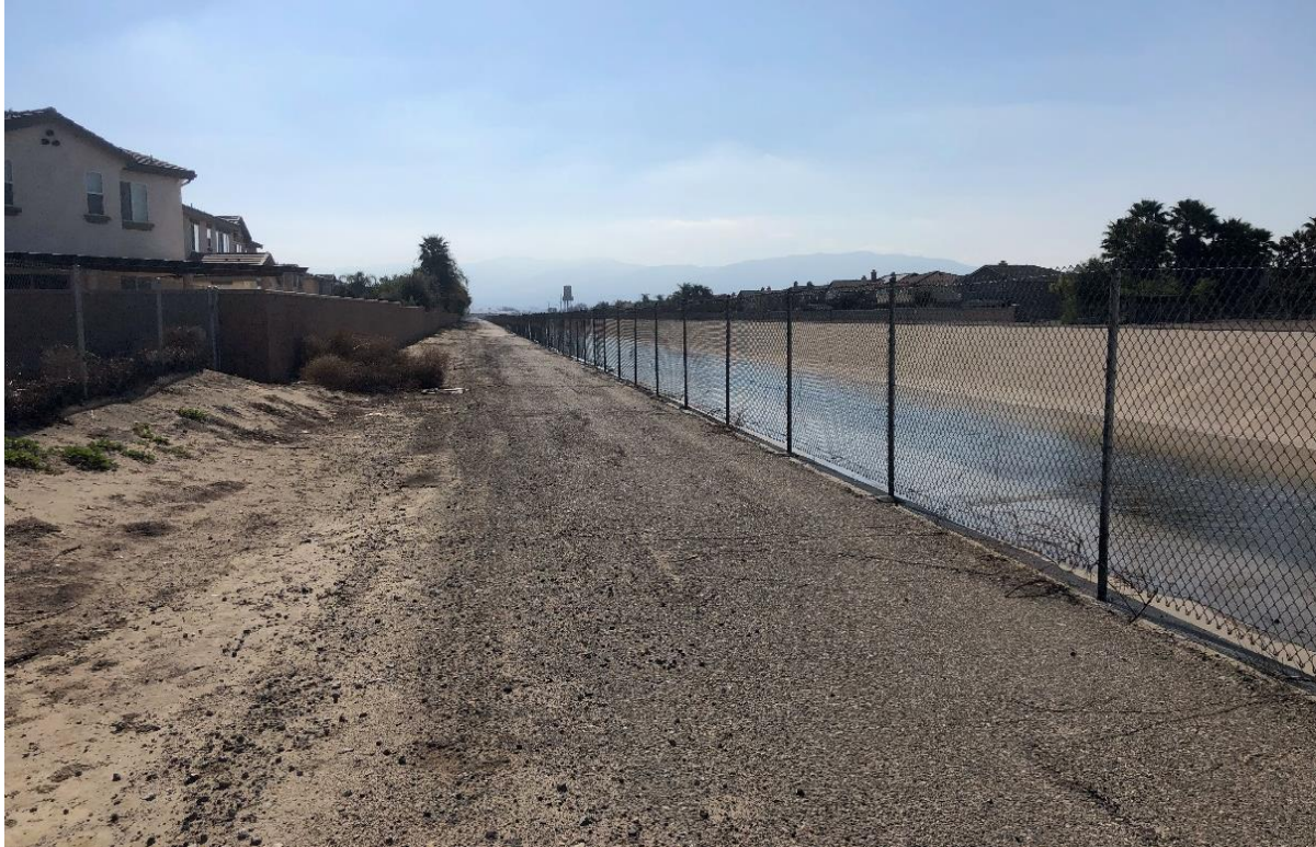
Photograph 7. Downstream Cucamonga Creek Channel from the eastern bank. View to the south.
